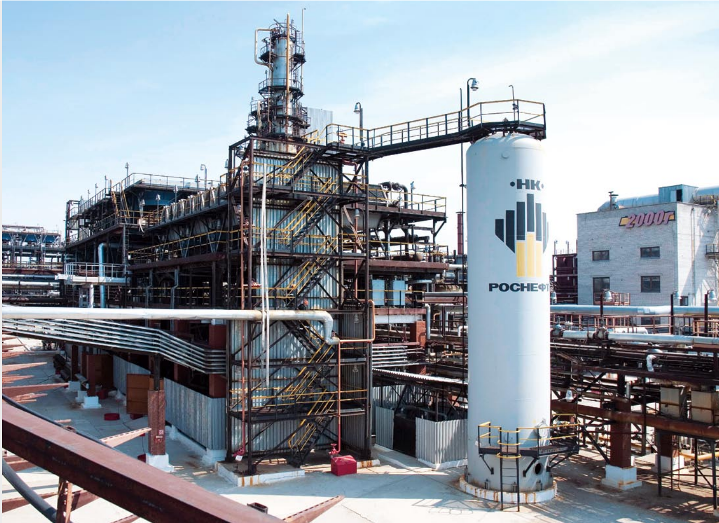
Catalytic reforming unit at Komsomolsk Refinery
